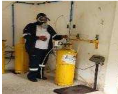
Excellent OHS at chlorine dosing facility at Bethulie WTW
