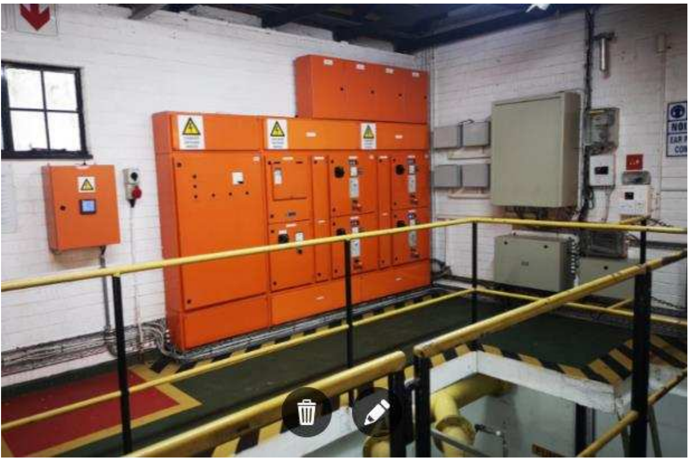
City of Johannesburg and Rand Water: Clean and well maintained pumpstation at Illovo Reservoir
