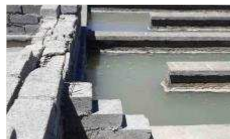
Flocculation channels walls poorly constructed and deteriorating
