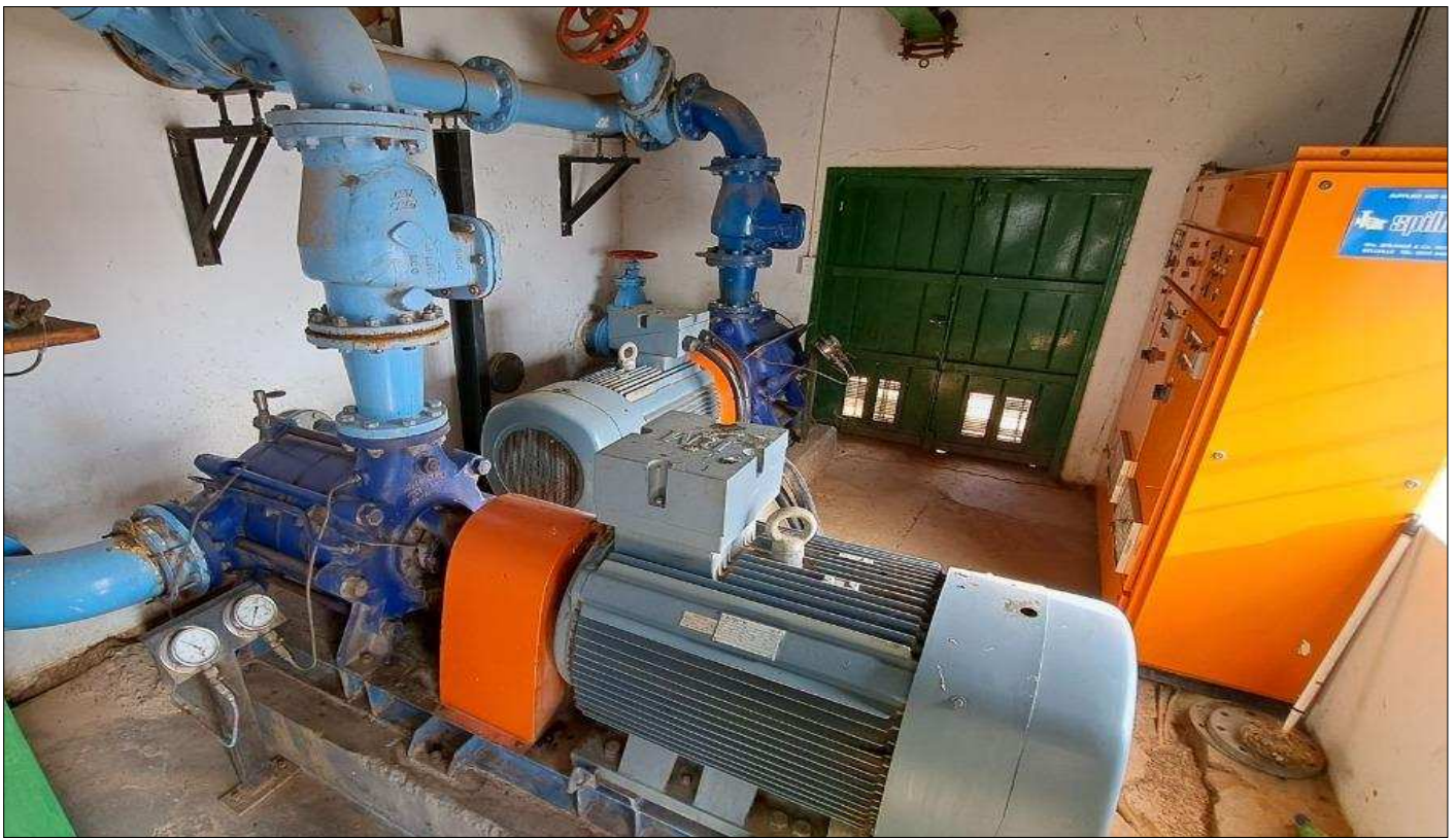
Bergriver: Piketberg WTW raw water pumpstation – deteriorating raw water quality, but staff displayed good knowledge of this risk via the water safety plan
