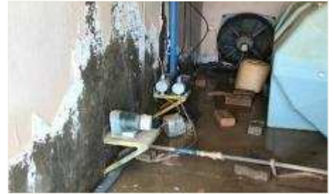
Deneysville WTW: Dysfunctional chloring dosing facility
