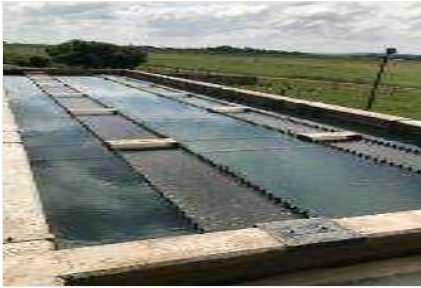
Deneysville WTW: Clarification
