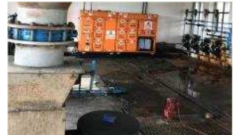
Chemical dosing area of the new WTW at Parys
