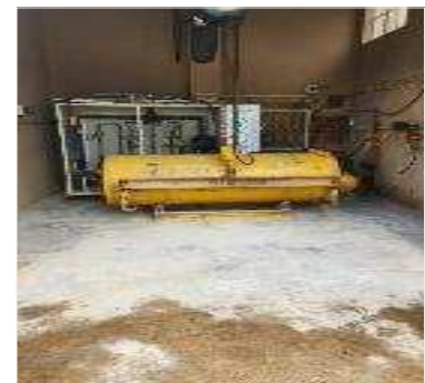
Poor chlorine dosing facility at Maselspoort WTW
