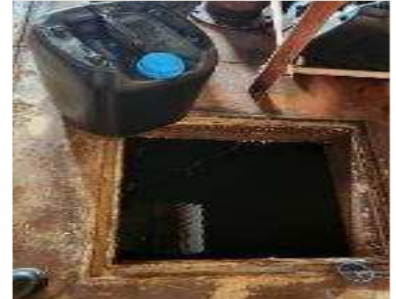
Final water sump is open, no method to control chlorine dosage at Winburg WTW
