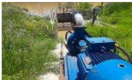
Raw water pump station at river, no standby
