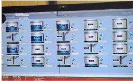
SCADA system at Balkfontein WTW
