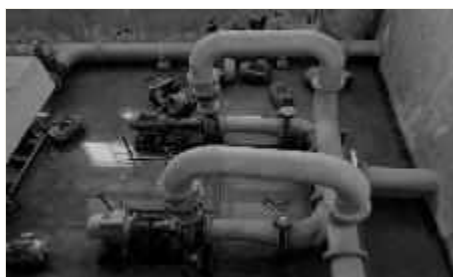
Highlift pumpstation floor under water
