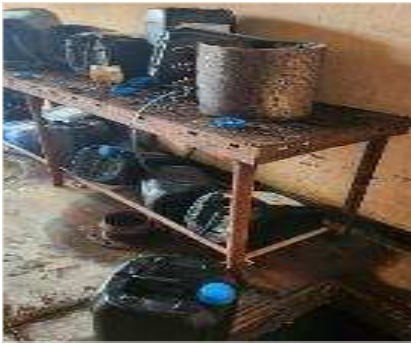
Open clear water tank on bottom left-hand side of picture, exposed to contaminants
