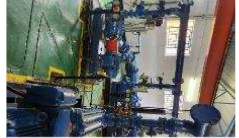
Final water pumpstation with duty standby pumps
