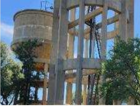
Matjhabeng high lift tower
