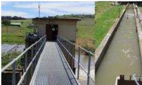
Raw water pump station abstracting from a weir in Wilge River. Accumulation of logs and debris during heavy rain. Flow measurement at inflow
