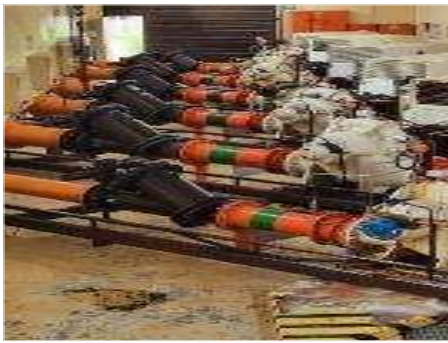
Final water pumpstation at Virginia WTW
