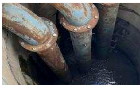
Raw water pump abstraction well from river. Poor OHS environment
