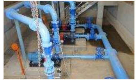
2 x pump sets pumping from clear water sump to large on-site concrete reservoir. Four pumps in high lift pump station, pumping from concrete reservoir to reservoirs in distribution
