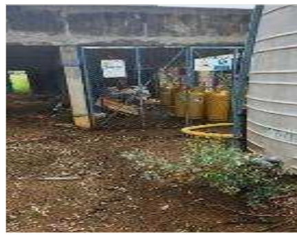
Chemical storage unit filled with rain and mud at Zastron WTW
