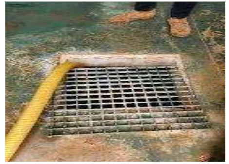
Clear water wells are uncovered to allow tankers to collect water at Zastron WTW
