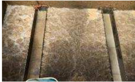
Deneysville WTW: Filter backwashing
