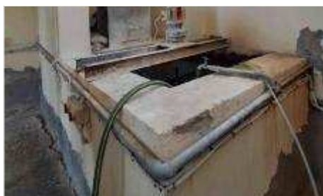
Lime dosing equipment in poor state
