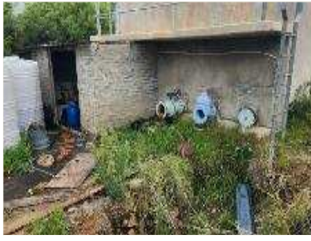
Terrain is covered with building rubble, old equipment, and huge holes
