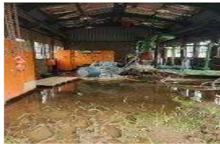
Final water pumpstation filled with mud and water, leaking pipes, no standby pump
