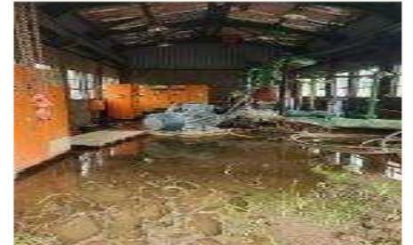
Final water pump station flooded at Genoa WTW
