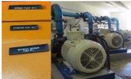
High lift pump station
