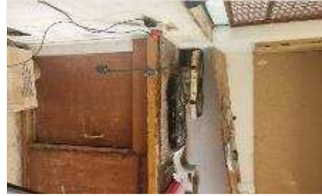
Poor staff facilities at Genoa WTW
