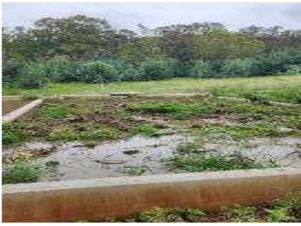
Sludge drying beds filled with sludge and weeds at Zastron WTW
