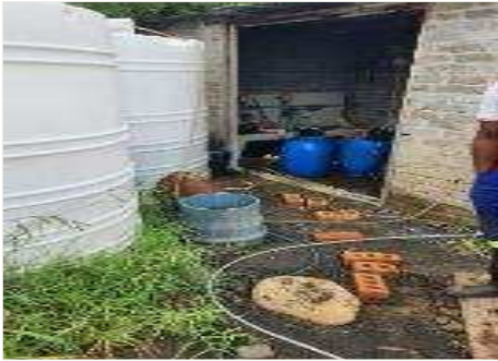
Poor state of chemical dosing room at Winburg WTW
