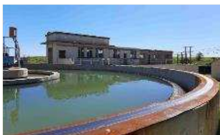
Top of clarifier wall where rotating bridge runs been covered with steel plate due to concrete spalling underneath
