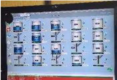
SCADA system at Balkfontein WTW
