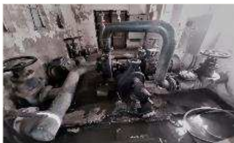
Main raw water pump station at the Dam
