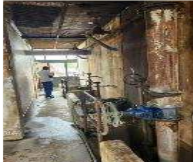
Filters in need of urgent upgrade at Winburg WTW
