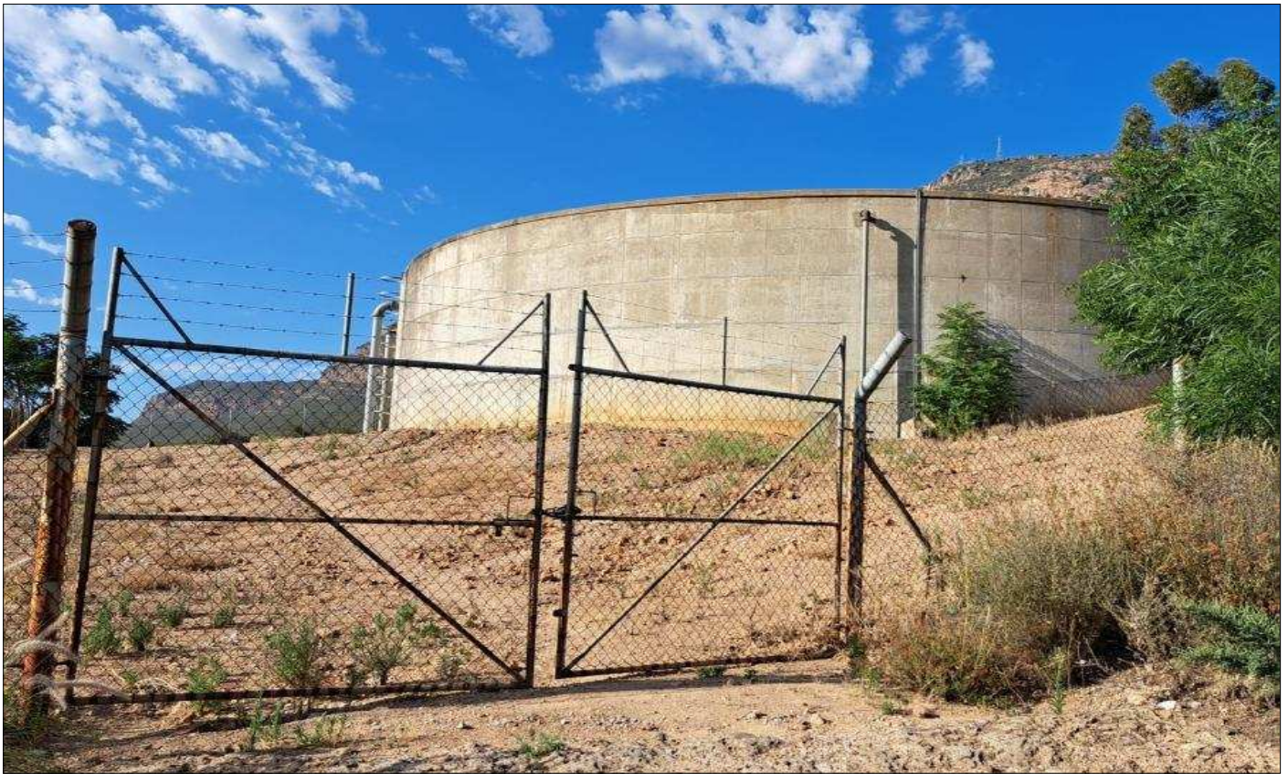
Piketberg reservoir secured with routine inspection regime
