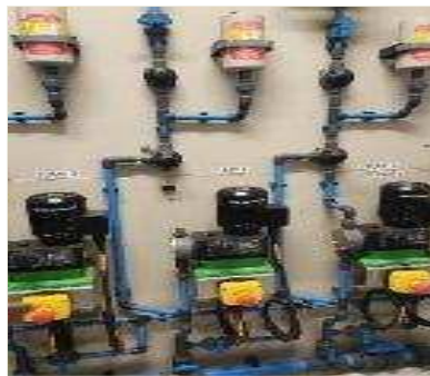
New chemical dosing facility at Maselspoort WTW
