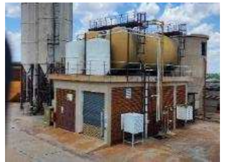
Bulk chemical storage at Balkfontein WTW
