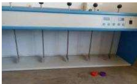
Picture of available six blade paddle stirrer at Hertzogville Water Purification Plant but not utilised
