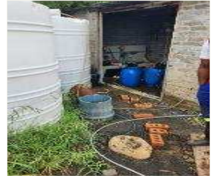
Chemical dosing facility has one dosing pump, no bunded walls around tanks and room filled with empty chemical drums
