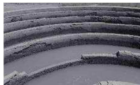
Circular flocculation channel in desperate need of refurbishment
