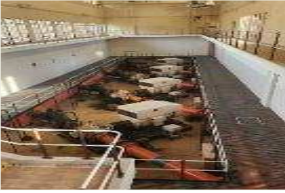
Final water pumpstation at Balkfontein WTW
