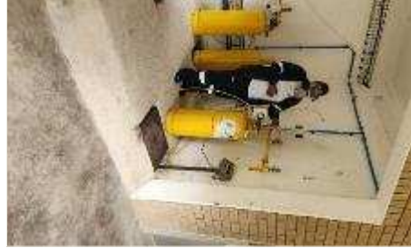
Good safety practice for chlorine handling at Bethulie WTW
