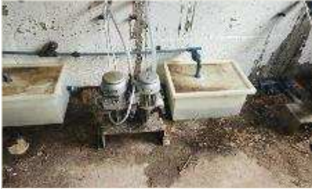
Chemical dosing room requires refurbishment, only one dosing pump, no bunded walls, no eyewash
