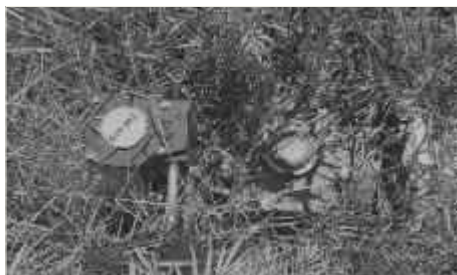
Final water outlet valve and meter (not working)
