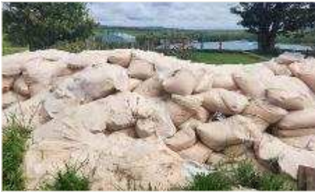
New filter sandbags which have broken open at Genoa WTW
