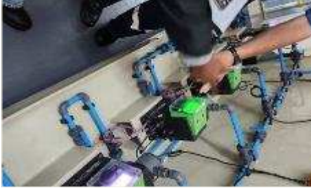
Duty standby chemical dosing p pumps at Bethulie WTW
