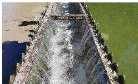
Launders within settling tank
